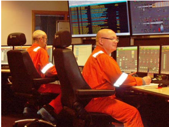
Central Control Room Operations
