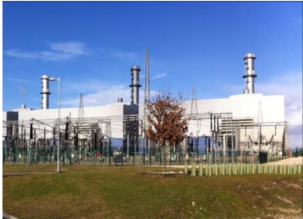
Switch yard connection to the National Grid
