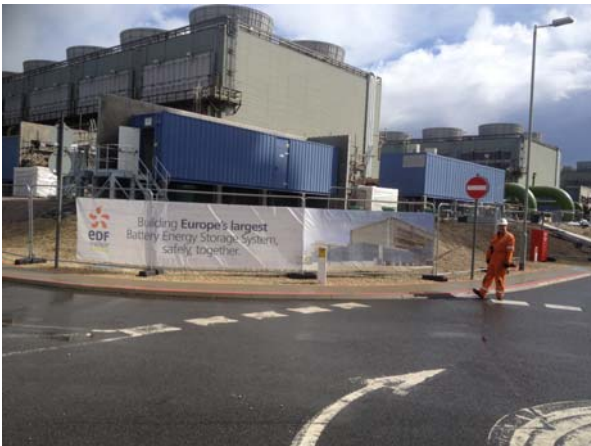
New Battery Energy Storage System
