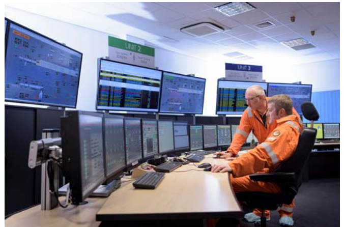
Central Control Room Operations
