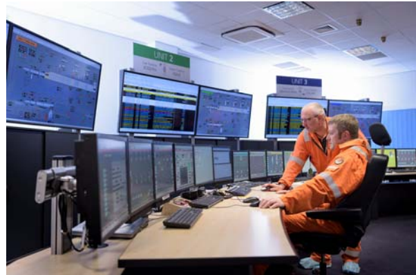
Central Control Room Operations
