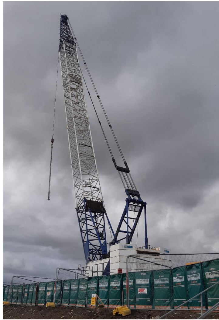
A crane is now positioned on the Abnormal Loads Quay to support the piling
