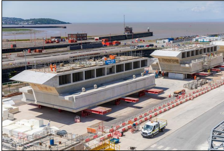
Figure A3-3 -Hinkley Point C’s LVSE intake heads are specially designed to reduce the speed at which water is fed into the cooling system
