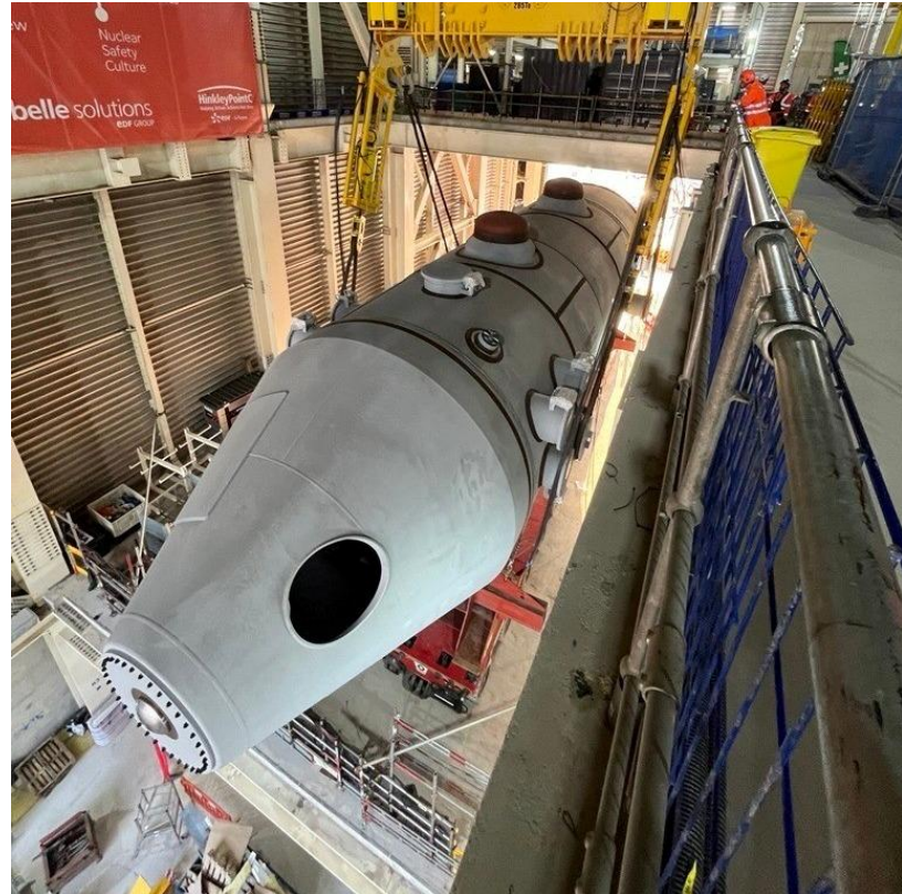
The 22-metre high MSRs were manoeuvred into place using the turbine hall's 300-tonne gantry crane.
